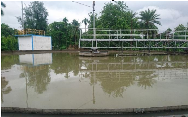
Sludge settling tank
